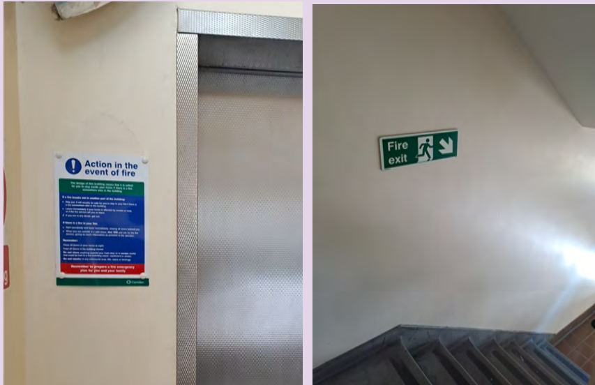
Fire Action Notice and Fire Exit Sign at 8 Newton Street.
