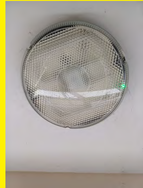
Emergency light at 8 Newton Street.
