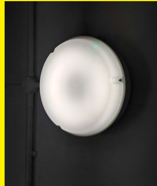
Emergency lighting at Great Russell Mansions.
