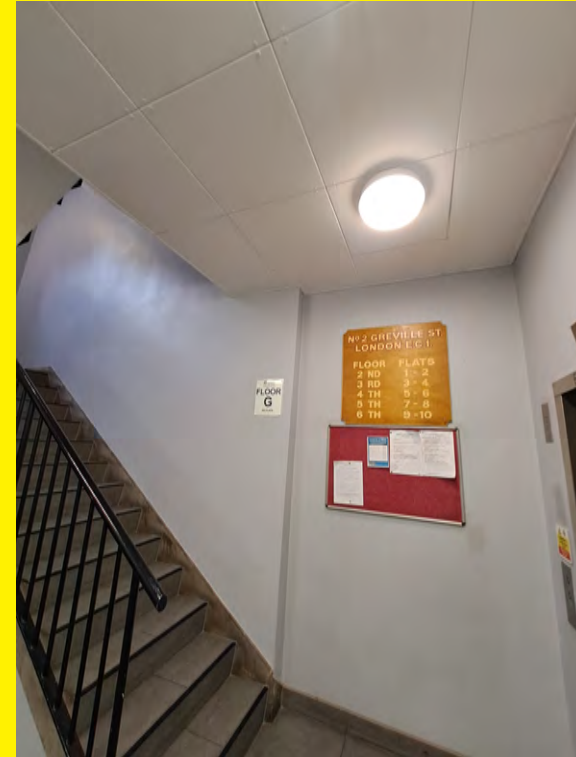
Emergency lighting in stairwell at 2 Greville Street.
