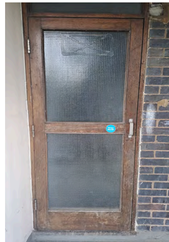
Internal staircase fire door at Barrington Court.
