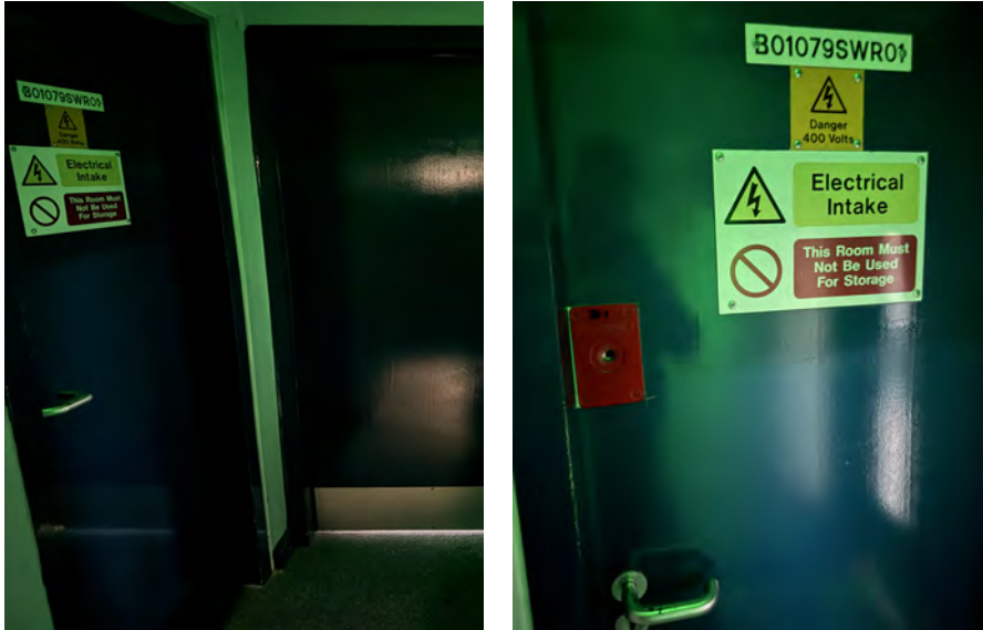
Electrical Intake Cupboard Fire Door at Barrington Court.
