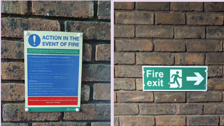
Fire Action Notice and Fire Exit Sign at Mayford.
