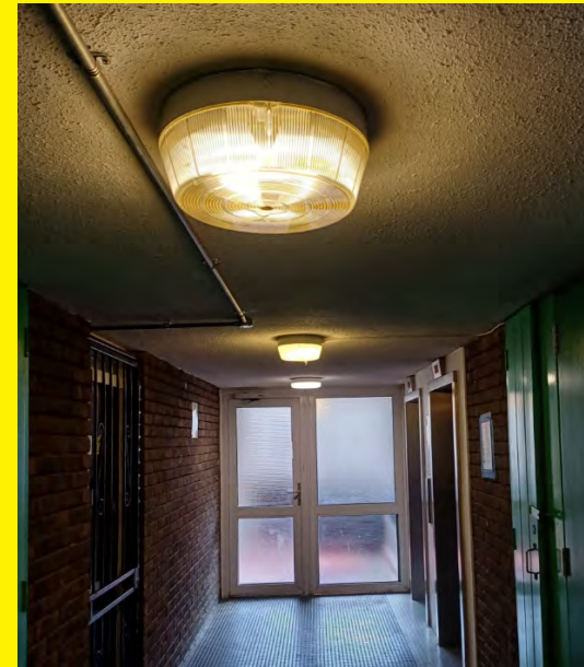
Emergency lighting at Mayford.
