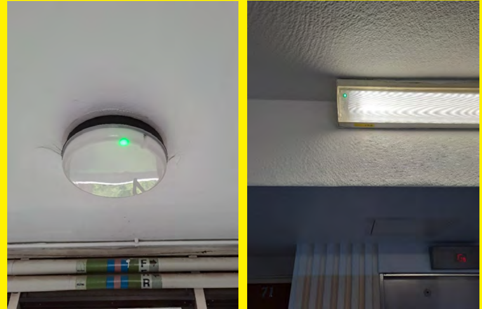
Various Emergency Lighting at Blashford Tower.
