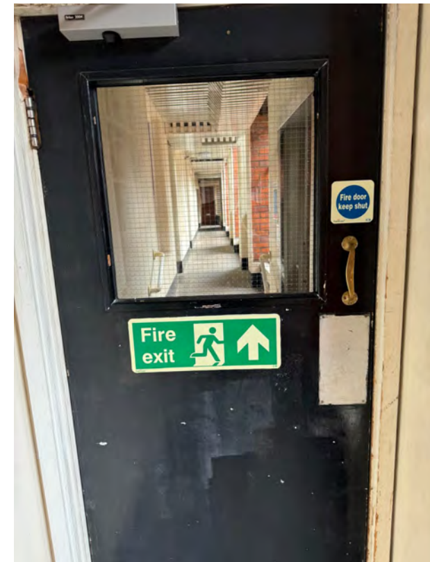
Communal Fire Door at Seymour House.
