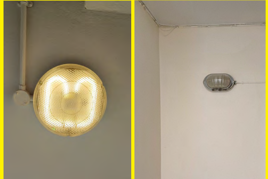
Emergency lighting at Hardington.
