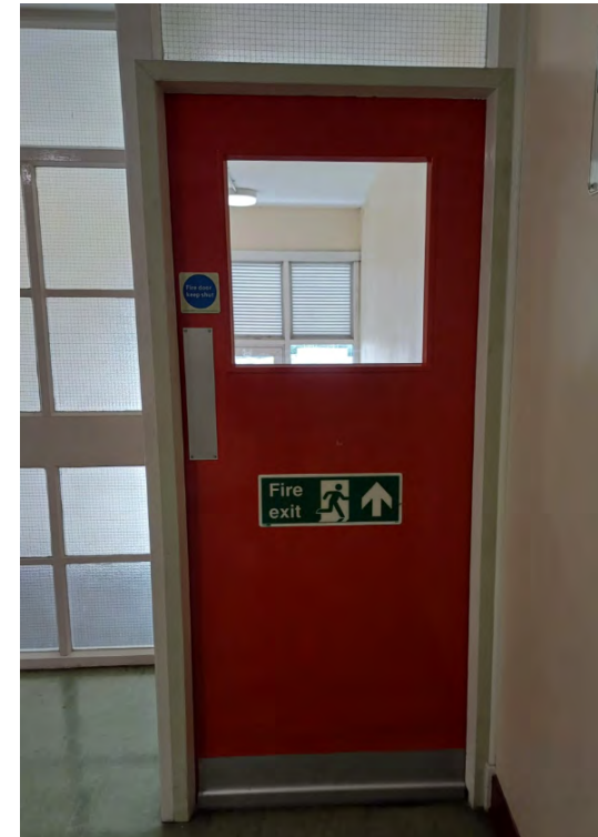
Communal Fire Door at Hardington.
