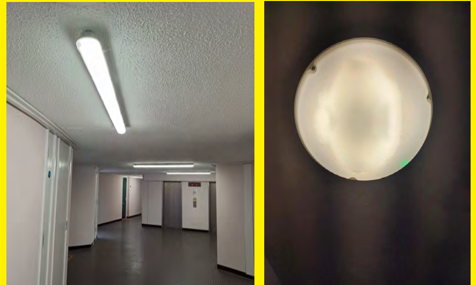
Emergency lighting at Jeygrove Court.
