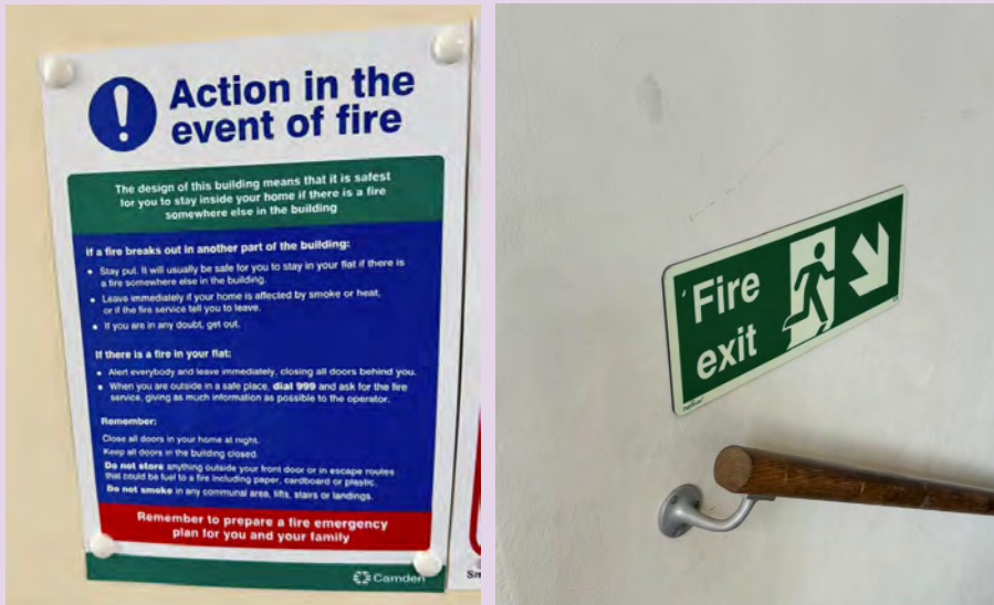
Fire Action Notice and Fire Exit Sign at 1-35 Hunter House.
