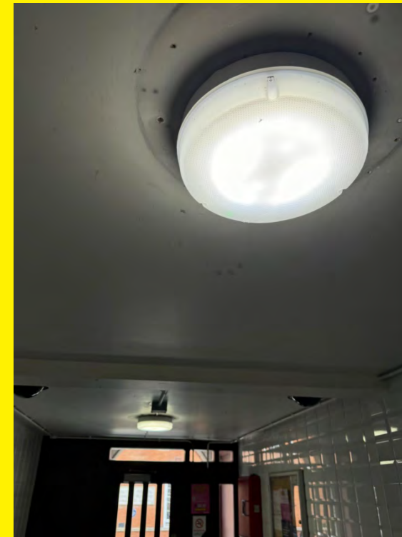
Emergency lighting at 1-35 Hunter House.
