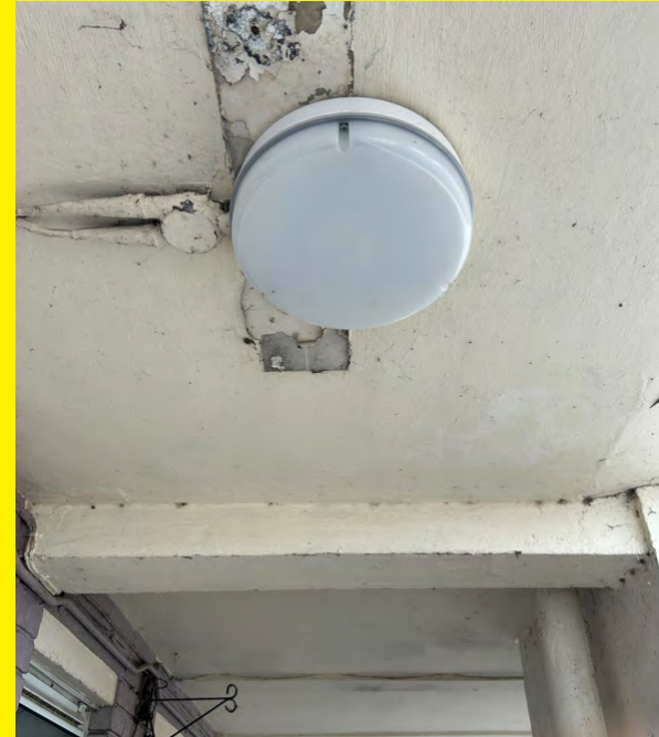
Emergency lighting at 1-28 Culver House.
