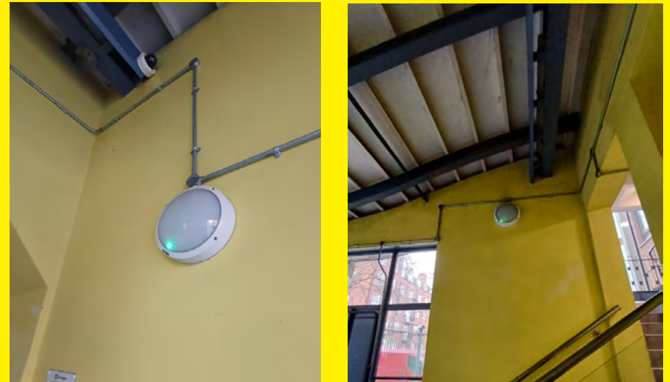
Emergency lighting at Hollisfield.
