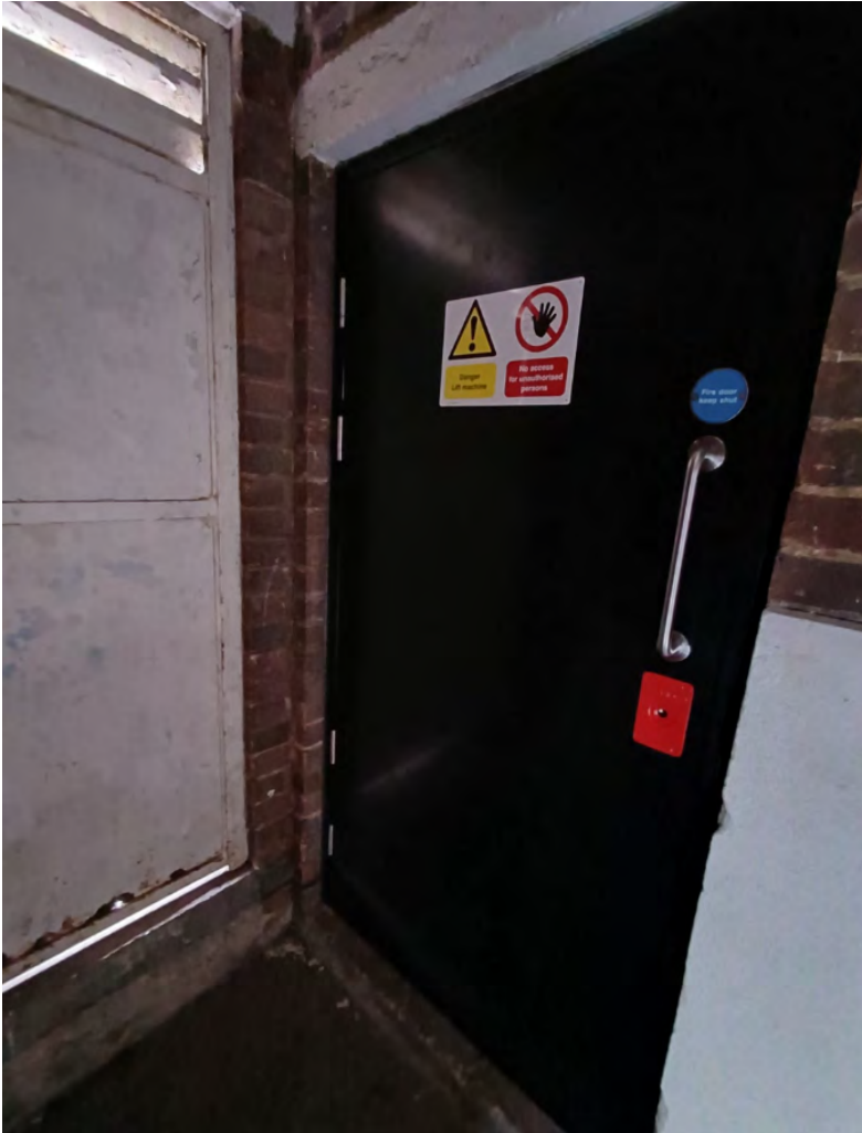
Lift Motor Room Fire Door at Hollisfield.
