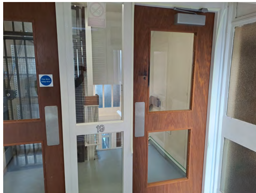
Communal Fire Doors at Snowman House.
