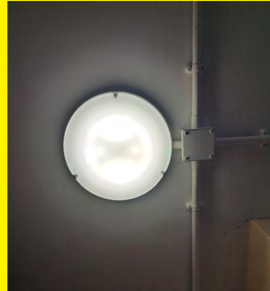
Emergency lighting at Snowman House.
