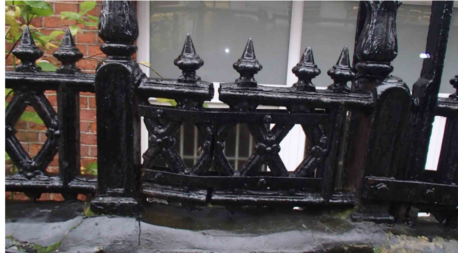
Damaged railing, 59-61 Hatton Garden
