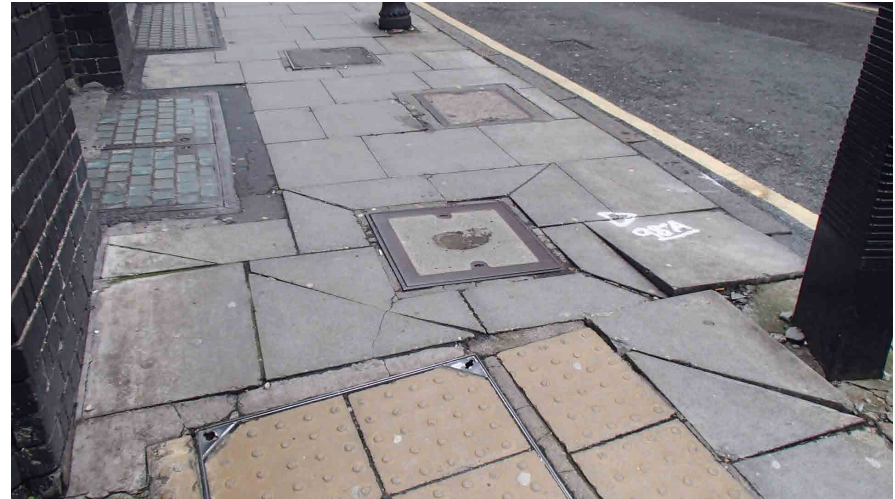
Poorly laid paving, but good quality granite curb stones, Greville Street
