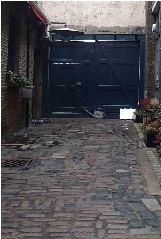
Badly re-laid granite setts, Bleeding Heart Yard
