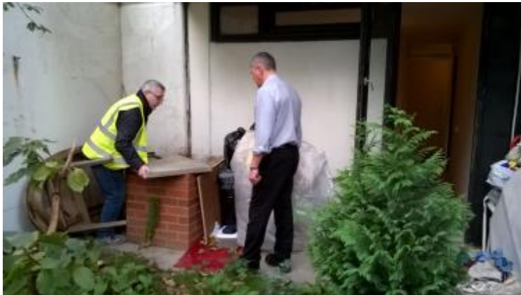
Connection to DH network. (External, above ground, not insulated)
