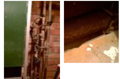
In-dwelling hot water storage + radiators
