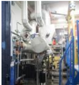
Central boiler room
