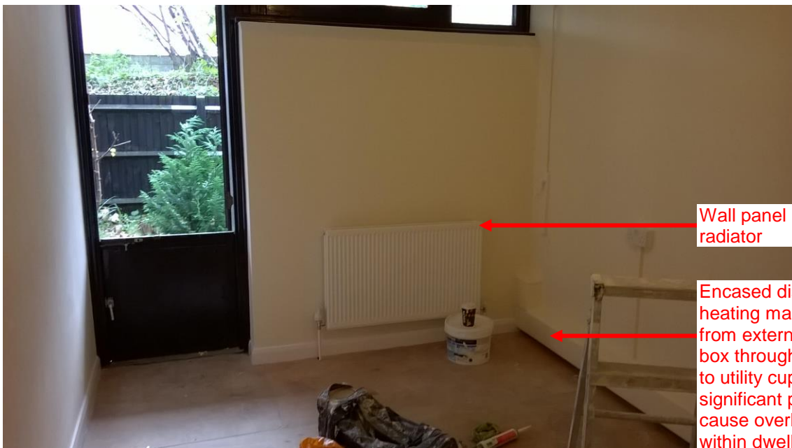
Wall panel radiators have been installed although residents have expressed their preference for trench radiators for future works when the district heating is updated
