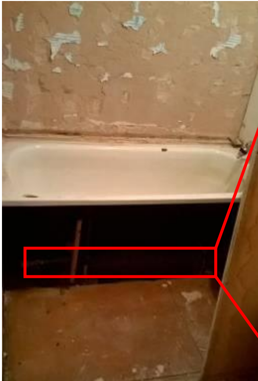
PHOTO B: Trench radiator and TRV (temperature control) located behind bath panel and thus completely inaccessible to resident, with overheating inevitable
