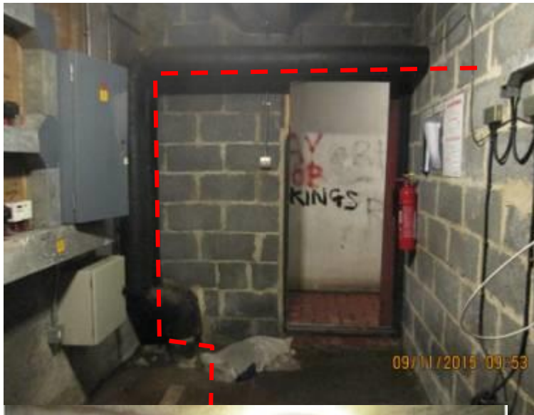
D. Network passing through basement storage areas
