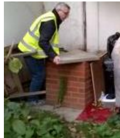
Branch connection at dwelling
